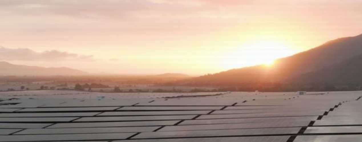
ACEN San Marcelino 383MWp Project Philippines' largest PV plant under construction Passed VRE Test in 2 days
